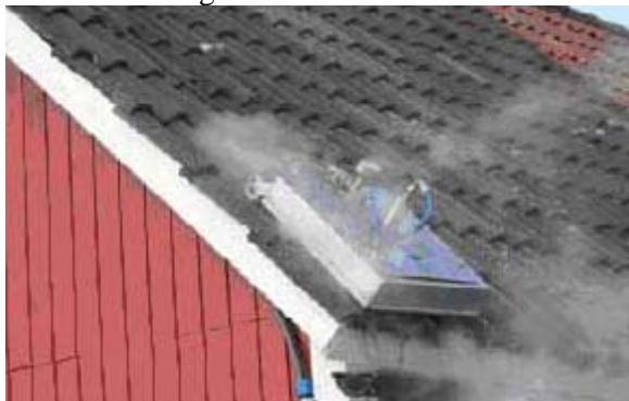
Fig 2. The hot water trolley at work on the concrete roofing tiles of the DEMOEX house.
