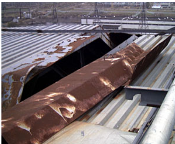
FIG. 6.3. Opening at the “Shelter” allowing infiltration of atmospheric water.
